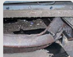
Missing predetermined breaking point
