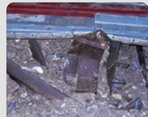
Missing predetermined breaking point
